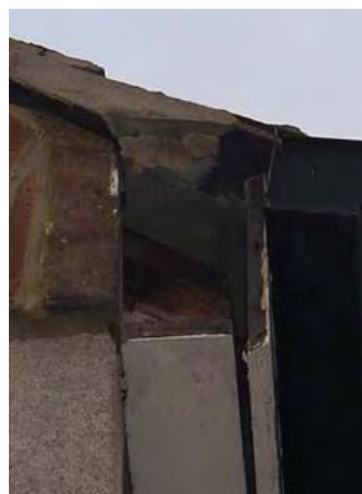
Figure 10 Gap in Soffit at South-Eastern Corner
