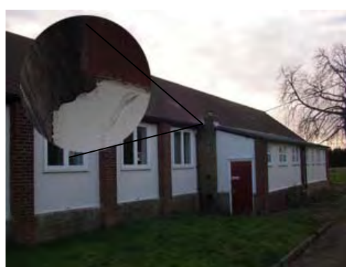
Figure 20 Boiler House with Potential Bat Access Gap
